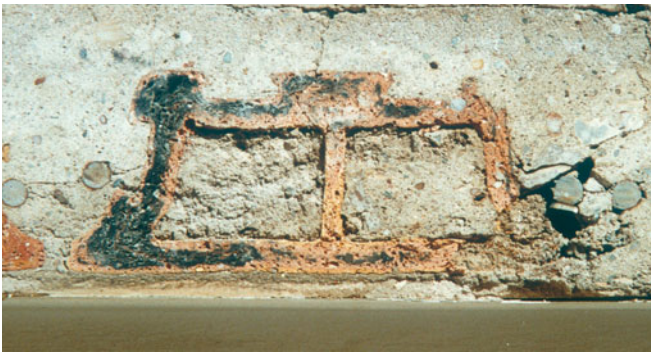
Typical cross section of a reinforced brick floor from about 1910, with brick, steel and concrete (Photo: Lorenz)
