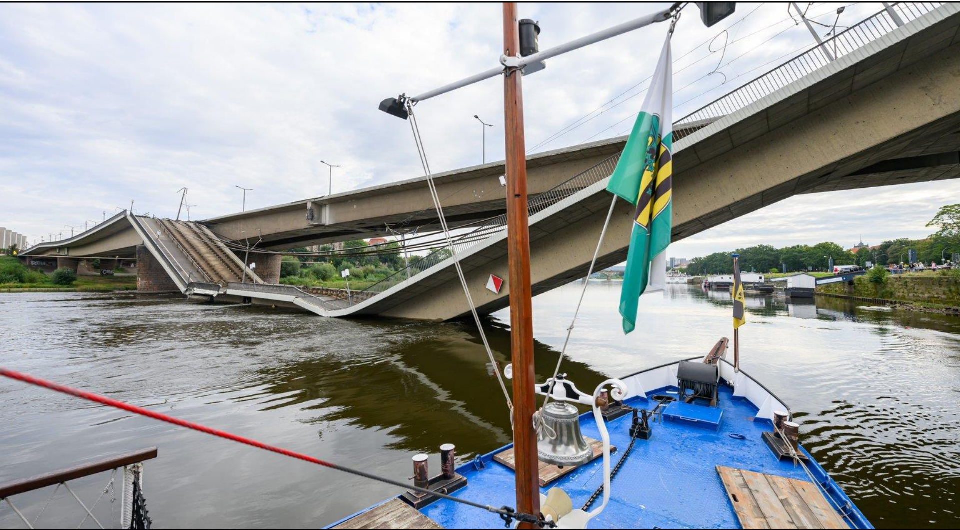
Dresden: Collapse of the Carola-Brücke on 11th September 2024 Photo: picture alliance/dpa/Robert Michael
