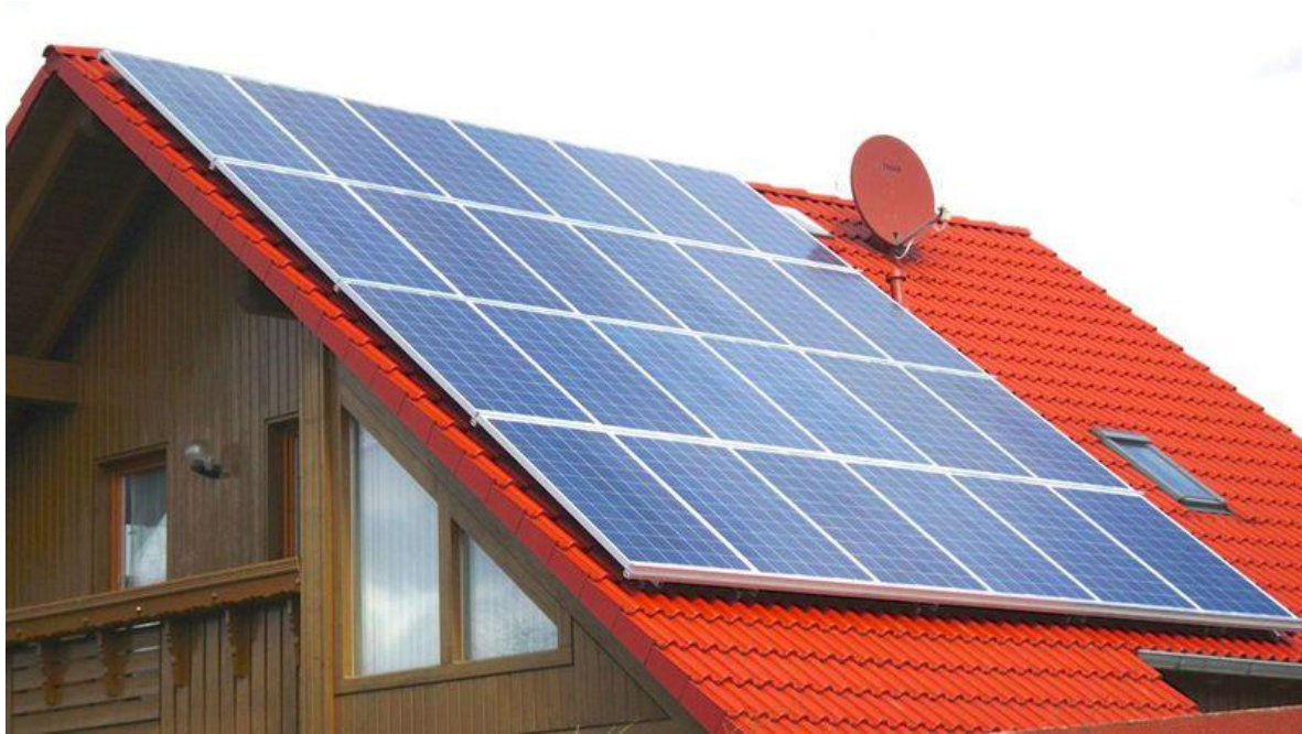
Fig. 2: Typical PV roof installation in local distribution grids
