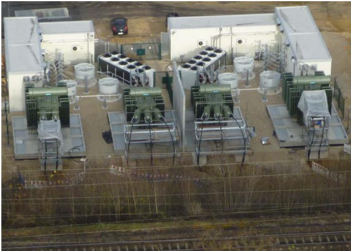
Fig. 3: railway converter, like it is placed near to the railway station Cottbus
