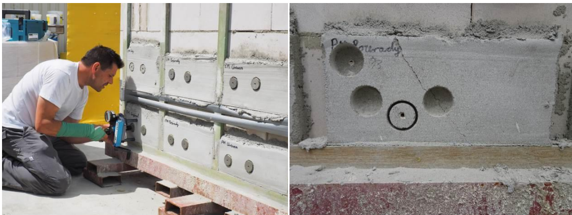
Fig. 8 – Test of bonding strength & detail of the compound mortar placed on a wall (photo: SAKRET Trockenbaustoffe Sachsen GmbH & Co. KG, Gewerbepark Diethensdorf 1, 09236 Claußnitz, Germany)
