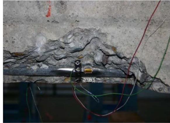
Fig. 6.9: Exposed area for determining the elongation of the prestressed steel under load
