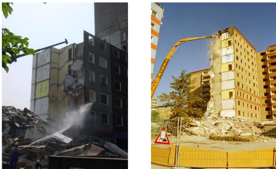
Fig. 3.16: Demolition of an 11-storey P2 type building by means of a hydraulic excavator and long front boom in Cottbus-Sachsendorf, 2003 (left); by means of a hydraulic excavator and demolition boom in Cottbus-Stadtring, 2007 (right)
