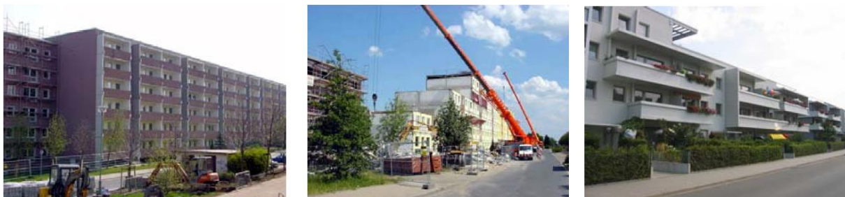
Fig. 3.15: Dresden-Gorbitz "Kräutersiedlung" 36 - old condition (left), interim status (middle), condition after dismantling (right)
